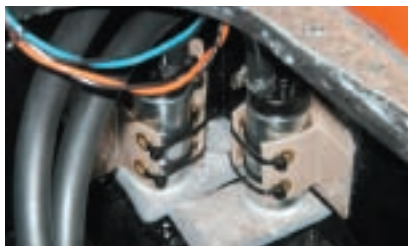
Built-in pump mounts for High & Low pressure fuel pumps.
